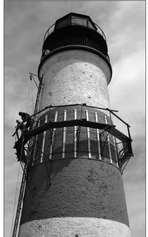
The spring crew from International Chimney Corp. work on the exterior bracing of the Lighthouse in May.
