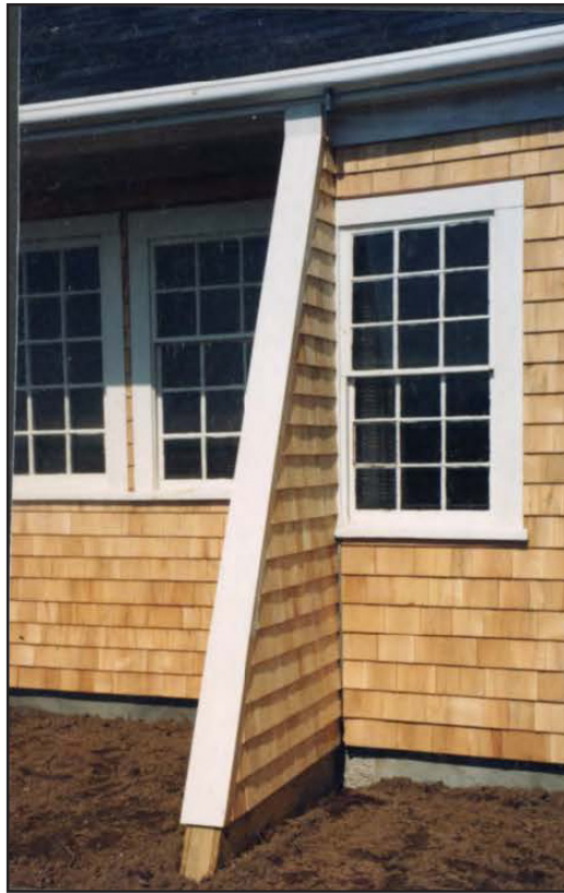
Heller O'Reilly Collection: Ca 1997 photo showing new buttress rebuilt to fit on new foundation with the elimination of the curve and woven shingle courses
